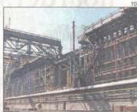
The newly-built coke oven battery of SAIL's IISCO Steel Plant
